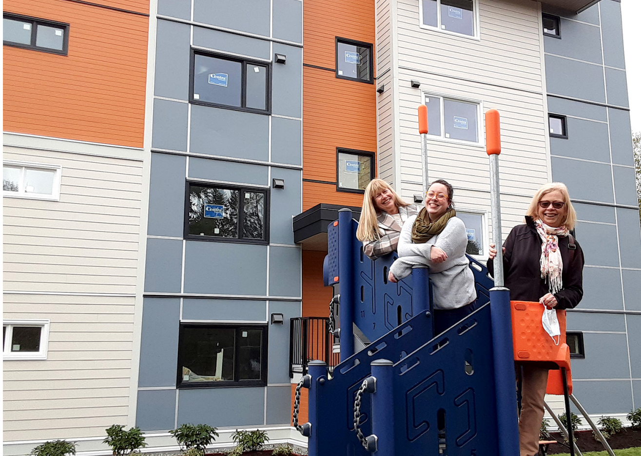
LADIES WHO LAUNCH: Still under construction, inclusion Powell River's new affordable housing building on Ontario will be ready for move-in January 1. On the playground are Louise Williams, BC Housing and developer liaison, Ceilidhe Maher, the contact for tenants; ; and inclusion CEO Lilla Tipton.
