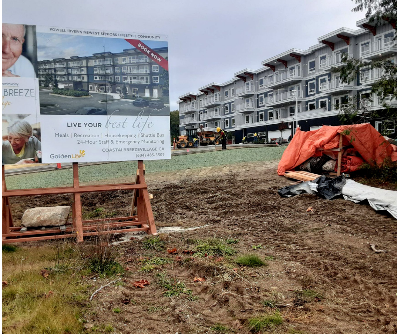
PART OF THE FIX: The 76 units of seniors rental housing at Coastal Breeze are nearing completion on Joyce Avenue. After a high in 2019, new residential development permits have waned.
